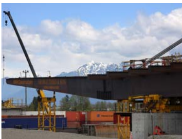
Hydraulic jacks of the 'launch system' push the girders with the 40m 'launching nose' at the front.
